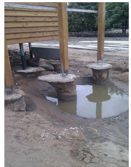
Footings scoured out by fast flowing water
